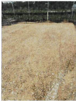
Figure 1: Transformer pad foundation.
