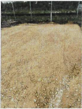
Figure 1: Transformer pad foundation.
