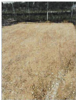
Figure 1: Transformer pad foundation.
